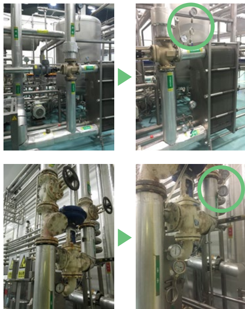
Installation of temperature and pressure gauge meters at inlet and outlet pipeline of PET line and sugar dissolving treatment at Luohe
