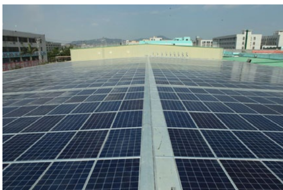
Photovoltaic panels at Luquan bottling plant in Mainland China
